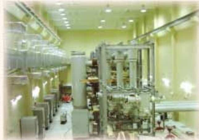
230 kV GIS Substation at Juaymah, Saudi Arabia
