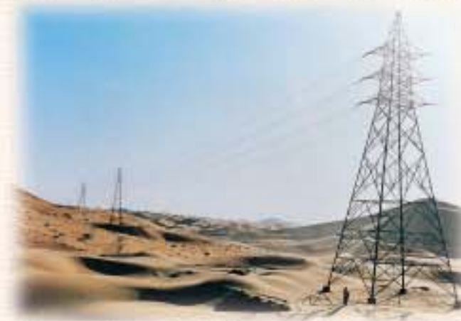
33 kV D/C Transmission Line at Abu Al Abiyad, UAE
