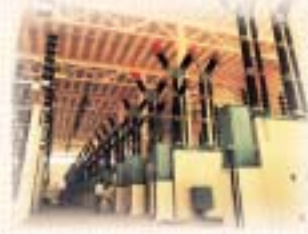
220 kV Indoor Substation at Tuticorin, India
