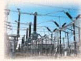
400 kV Switchyard at Uppal, India
