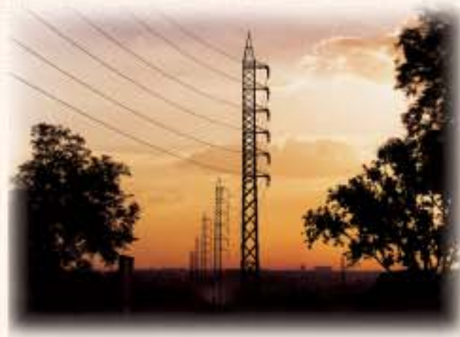
66 kV D/C Narrow Base Towers, Karnataka, India
