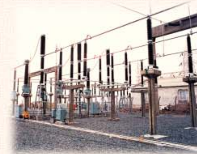
230 kV Switchyard with Pre-Stressed Concrete Supports, Tadipatri, India
