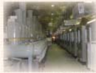
115 kV GIS Substation, Saudi Arabia
