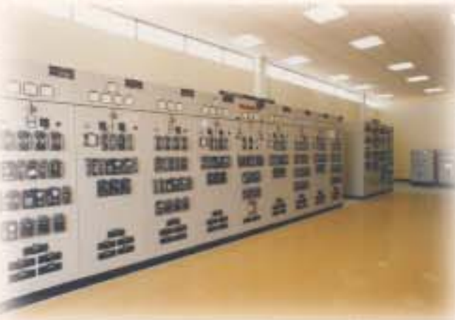
33 kV RCP at Ras Al Khaimah, UAE
